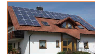
Off-grid home solar system
