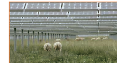
Farm solar generation system
